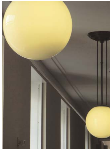
Refurbished Charles Holden light fixtures
